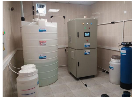
Aqua Park and Swimming Pool Water Disinfection Tehran Medical University Swimming Pool - 2019 Capacity: 6 kg FAC/d
